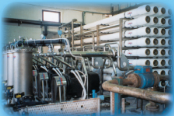
MUNICIPALITY CAPACITY: 2000 m 3 /day FEED WATER QUALITY: SEA WATER PRODUCT WATER QUALITY: POTABLE
