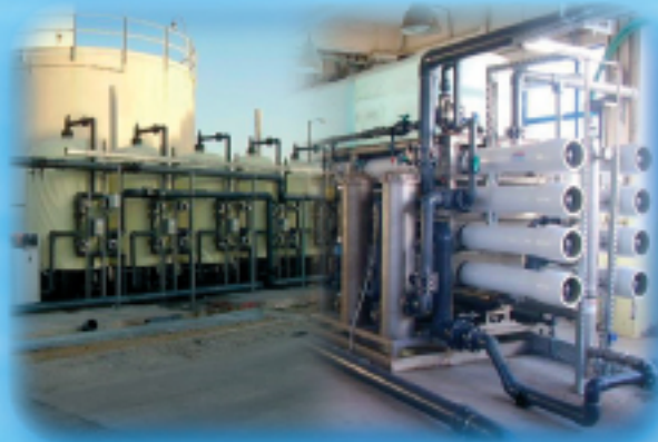
POWER PLANT CAPACITY: 960 m 3 /day FEED WATER QUALITY: SEA WATER PRODUCT WATER QUALITY: 300µS/cm
