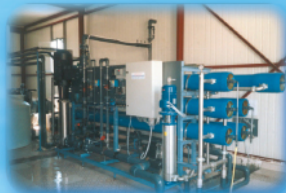
HOTEL CAPACITY: 700 m 3 /day FEED WATER QUALITY: 4000 - 7000 ppm TDS PRODUCT WATER QUALITY: POTABLE
