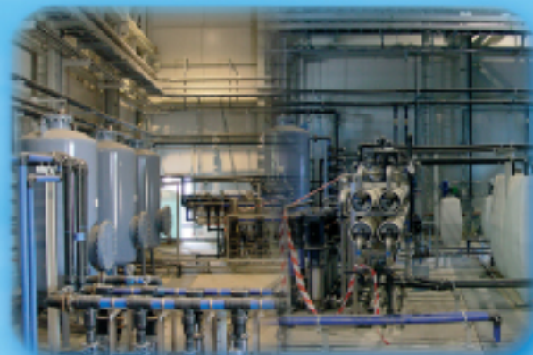
POWER PLANT – RO with Electrodeionization System (CEDI) CAPACITY: (2 x 243) m 3 /day FEED WATER QUALITY: BRACKISH WATER PRODUCT WATER QUALITY: ULTRAPURE WATER TO FEED BOILERS
